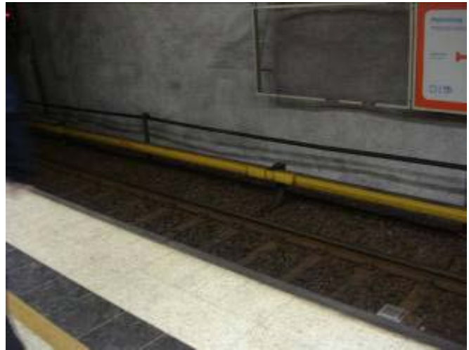
Figure 2. Yellow conductor rail at metro station
